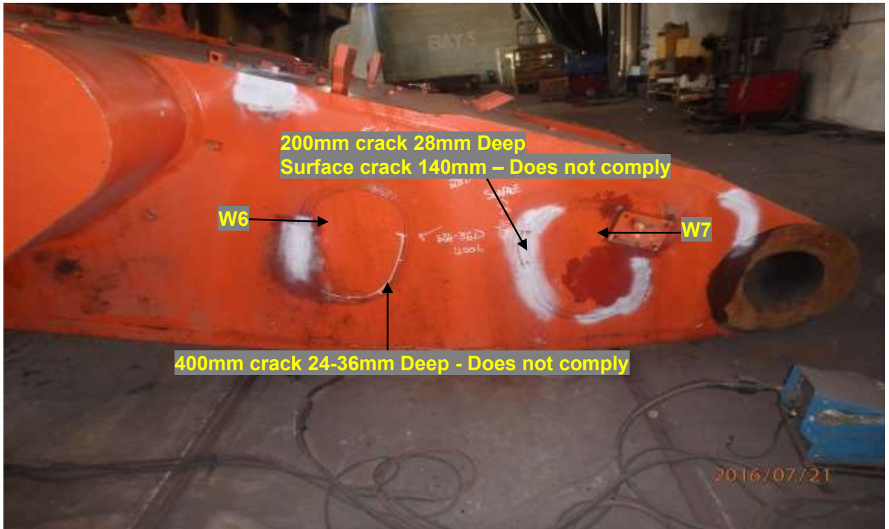
Photograph 1.3. General view of areas examined and discontinuities detected about EX5500 Boom.
