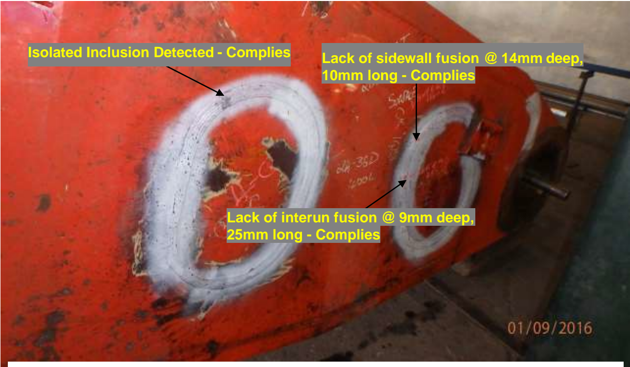
Photograph 1.2. General view of areas examined about W6 and W7 Windows, EX5500 Boom.
