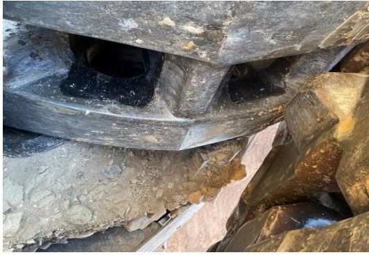
Figure 3 - Typical crawler shoe drive lug condition
