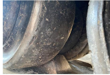
Figure 6 - LHS & RHS Rollers
