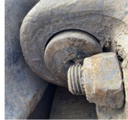
Pin / bore condition
